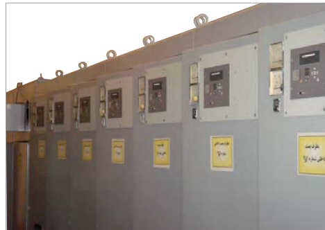
SIL-A relays installed in Azadi Football Stadium's electrical substation.
