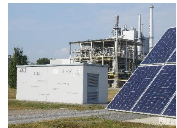
Prototype of a large lithium-ion storage system of the Energy Lab 2.0. (Photo: Battery Technical Center, KIT)
