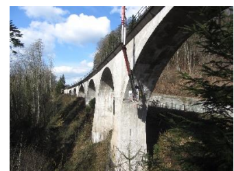
From a mobile platform underneath the Laufenmühle viaduct near Welzheim, radar and ultrasonic measurements were made. (Photo: KIT Innovation HUB)
