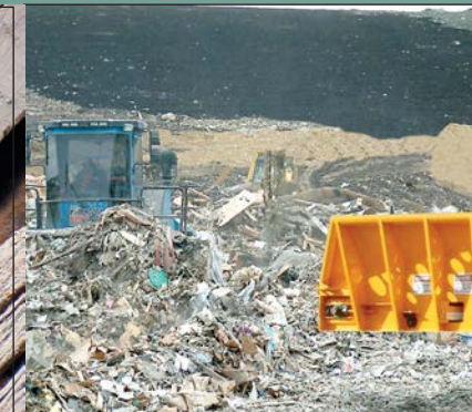
Grind ties with metal plates or contaminated C&D with the solid steel rotor and C&D screen
