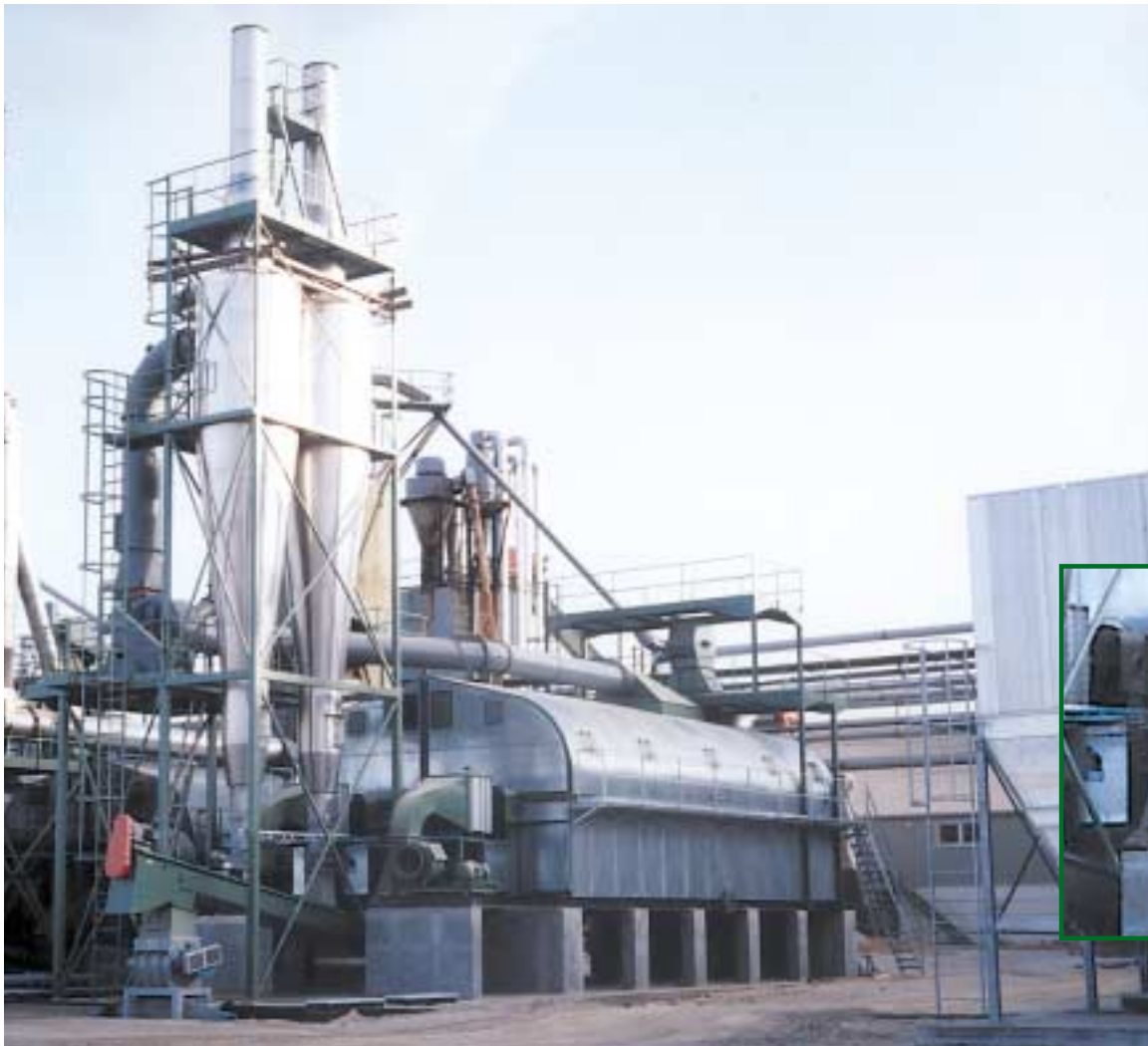
Chip drier with hot air injection
